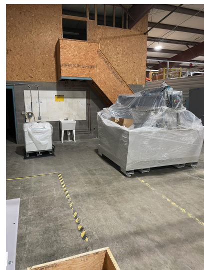
FLOW water jet to be installed in February of 2024.
